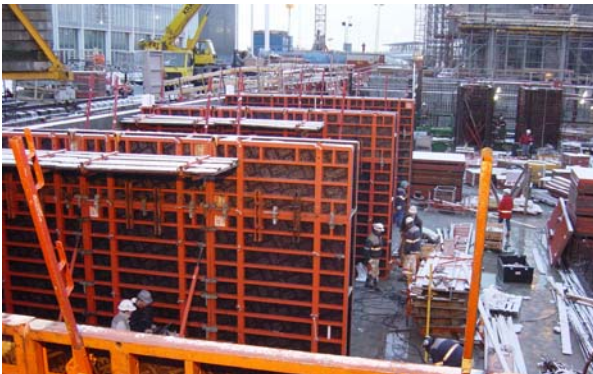
Ready for casting the three first walls of the basement with SCC, DR-Byen, Segment 3.
